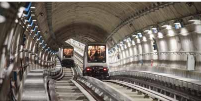
Automatic metro system in Turin – Lots 3 and 5 – Collegno-Porta Nuova section (tunnel length 5.3 km)
