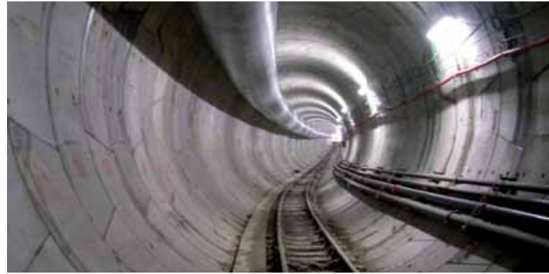
Naples metro system: construction of Dante-Garibaldi section, depot and workshop in Secondigliano, Piazza Dante station and Montesano corridor - Line 1
