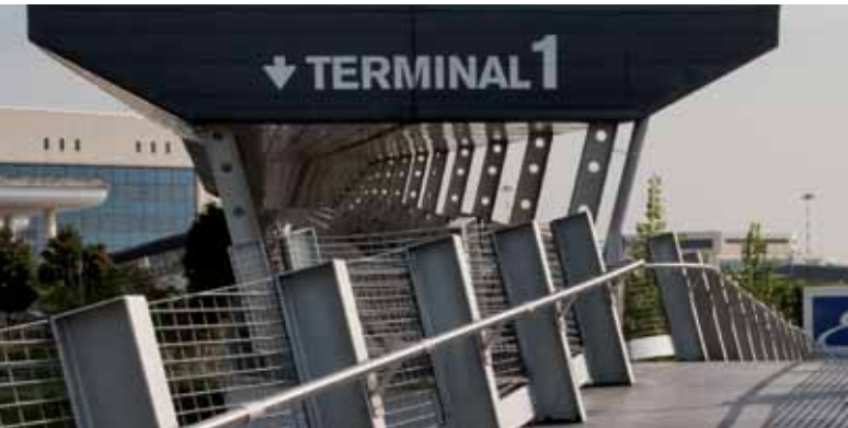
Milan Malpensa Airport: Completion of underground structures and construction of connecting walkway
